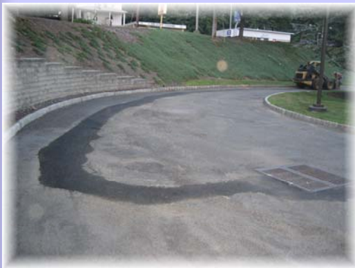
Drive Thru After Drainage Tile Installation To Redirect Water Away From The Retaining Wall
